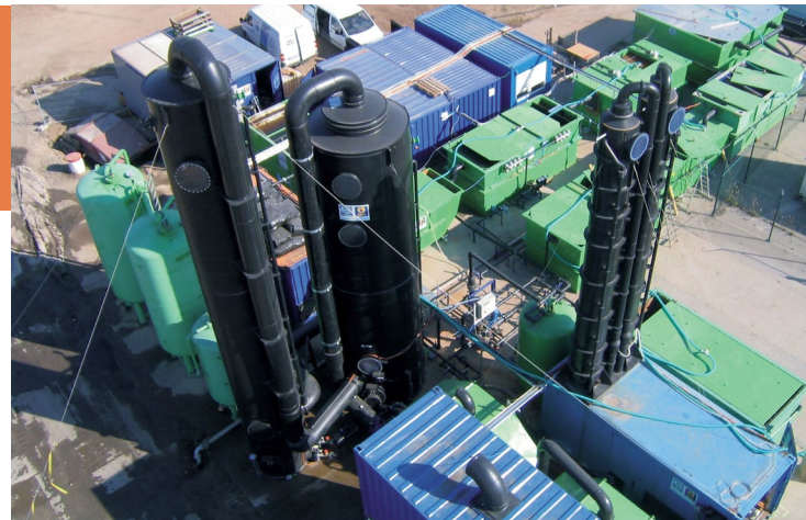
View of the groundwater treatment plant at Project Leuna.
