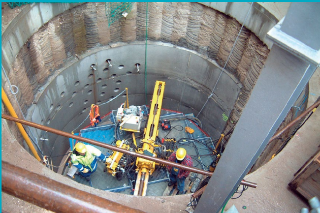
Auxiliary pit for the compensation grouting under existing buildings at the City Tunnel, Leipzig
