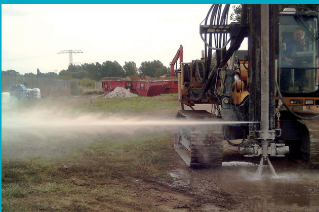
Cut-off wall for a major ecological water treatment project of the Leuna-Werke near Merseburg, Germany
