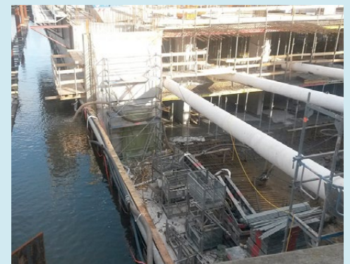
Excavation pit at the Hamburg Brooktor harbor for the extension of the corporate headquarters of Gebr. Heinemann.
