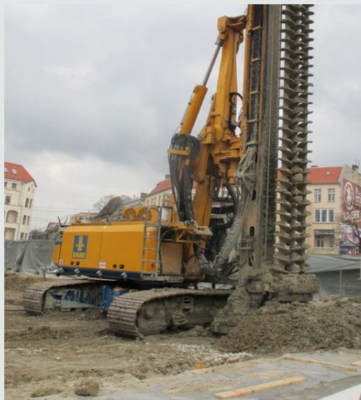
The MIP procedure has successfully been implemented at Wisbyer Straße in Berlin.
