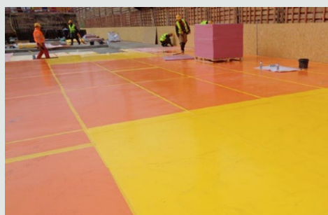
Elastomer mats are supposed to prevent vibration through railway traffic.
