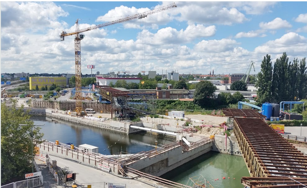
Construction site of the 16th construction unit of BAB A100 in the summer of 2016 at the Neukölln junction.
